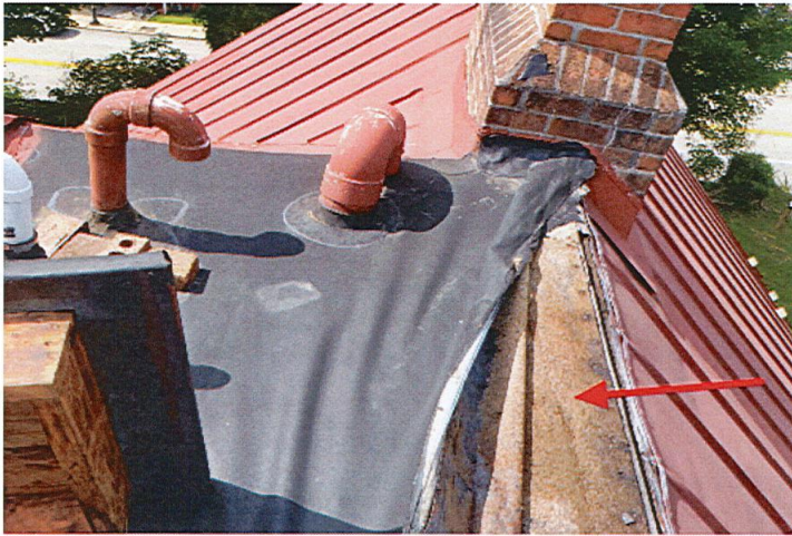
Rubber membrane is pulled away and leaving the iso board exposed. This is leaking now.
